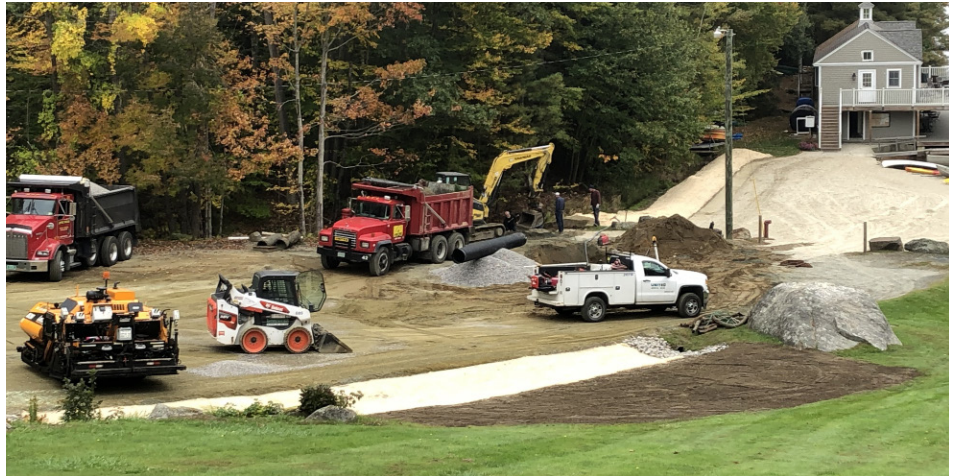
Construction underway at the Granliden erosion control project site, thanks to our partnership with the Granliden Community Association, Stone Environmental and United Construction. Photo by Becky Rylander.
