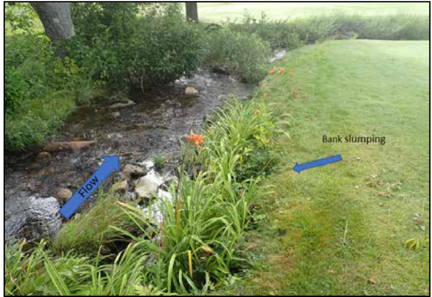
The slumping bank of this section of Kidder Brook will be stabilized with shoreline plantings.
