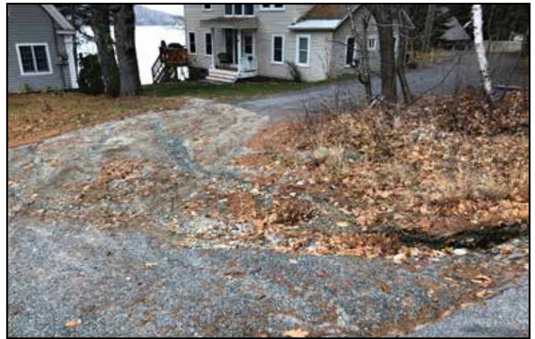
This erosion across a shared driveway will be addressed with a swale and infiltration trench.
